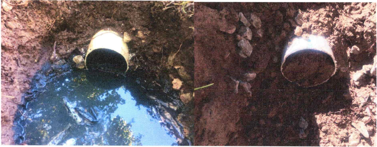
Figure 8 Discharge after cutting the end off a drain line
