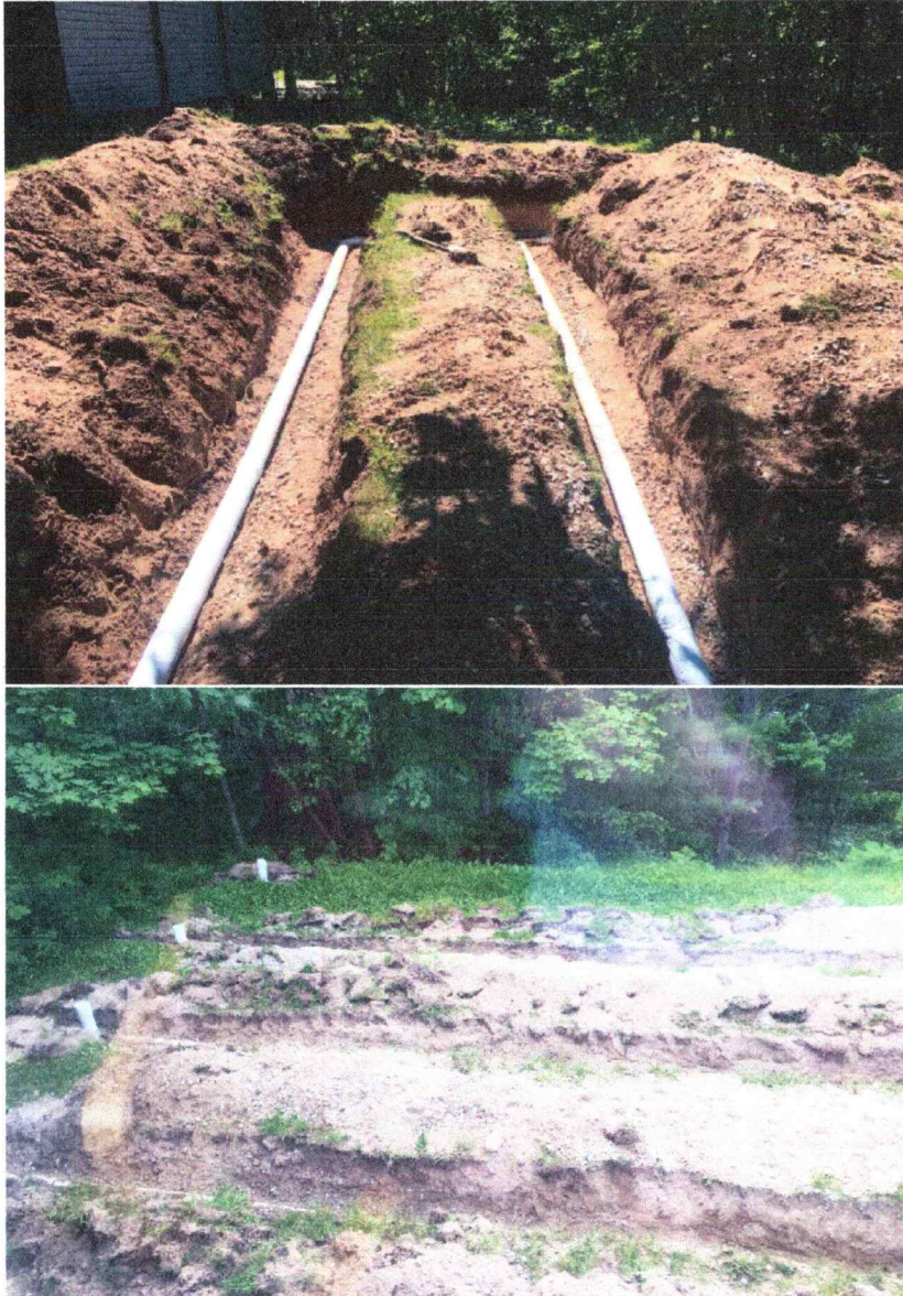
Figure 10 New Drain pipes the white pipes pointing up at the ends are observation pipes, used to get access for pumping or adding bacteria if needed.
